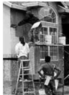
Workers unprotected from falling objects
